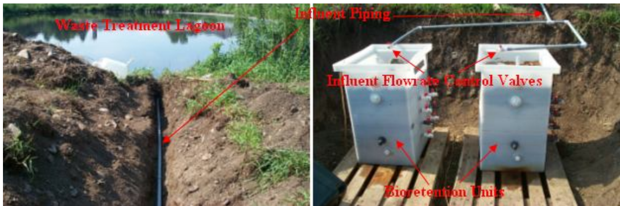
Figure 3.5: Influent Piping Layout during Field Testing of Bioretention Units
