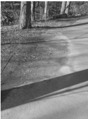
Figure 5. Conventional Off-Trail Raingarden Site Condition
