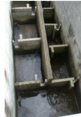
Fishway with notches and bottom orifices at Nunes mini-hydroelectric power plant
