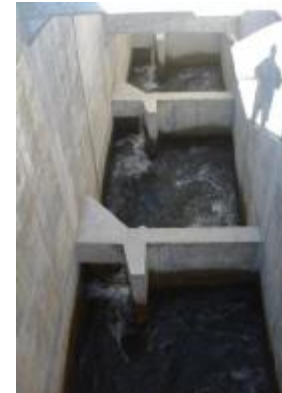
VSF at Açude-Ponte Coimbra
