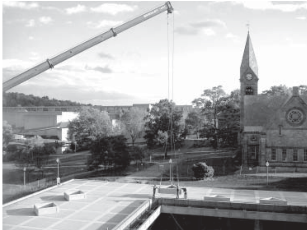
The new Du Bois Library plaza is in, there's a brand new beautiful entrance to the building, the trees will be planted in the planters come spring.
