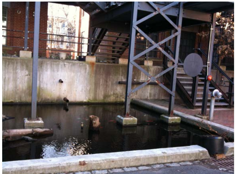
Rainwater harvesting pond. Source: M. Iarossi
