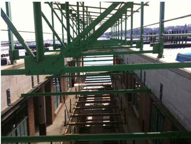
This building was cut in half, with the roof removed in the middle to allow more daylighting and better airflow.
