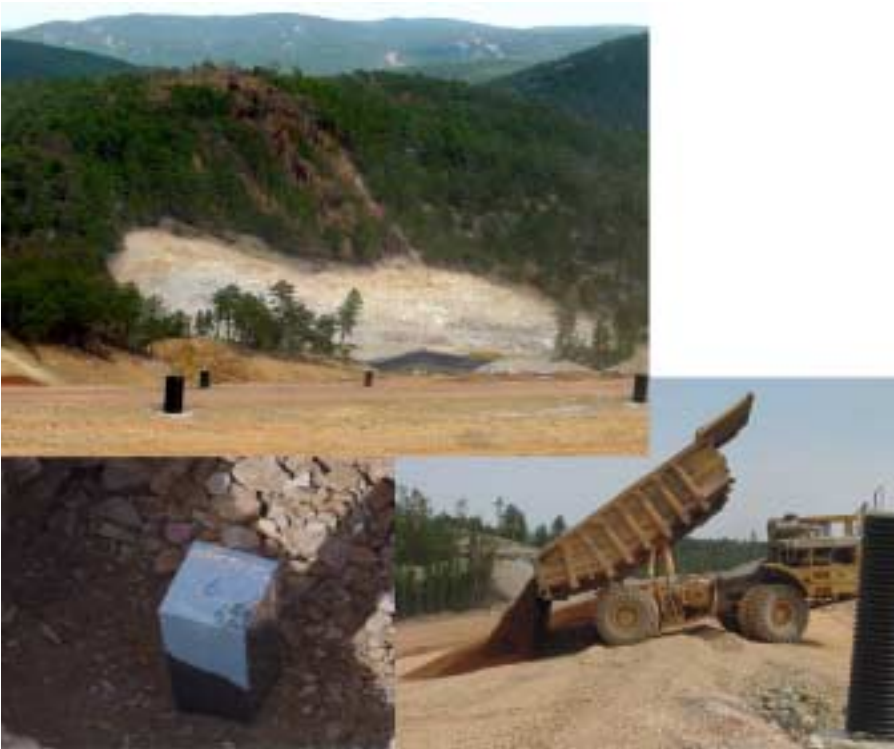
Figure 6. INL wireless sensor platform field test at superfund site in South Dakota.
