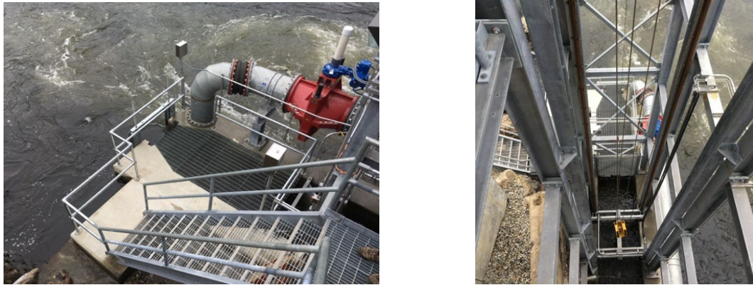
Figure 9. Scotland Fish Lift Tower (right) and fishway entrance (left) Image Credit: Brett Towler
