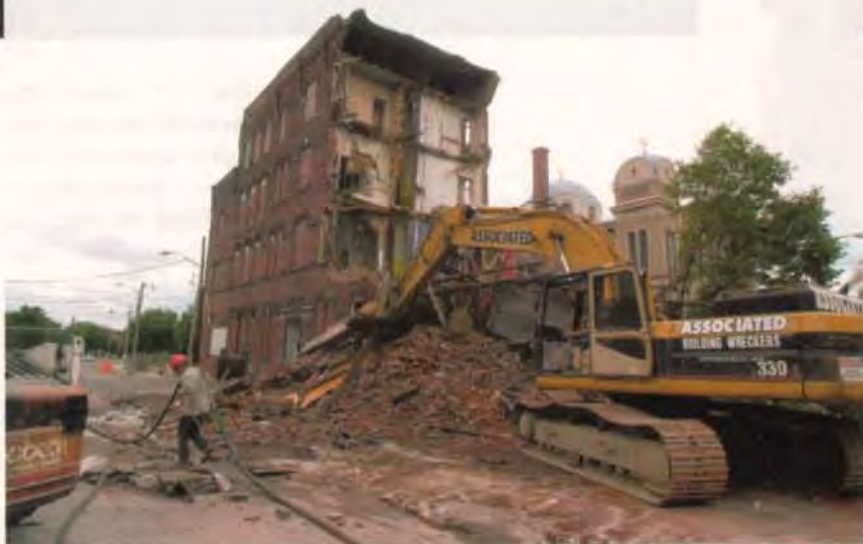
Despite a four-month reprieve and a desperate battle to raise money to renovate the Skinner building, the bulldozers and backhoes ultimately rolled in May 2006.
