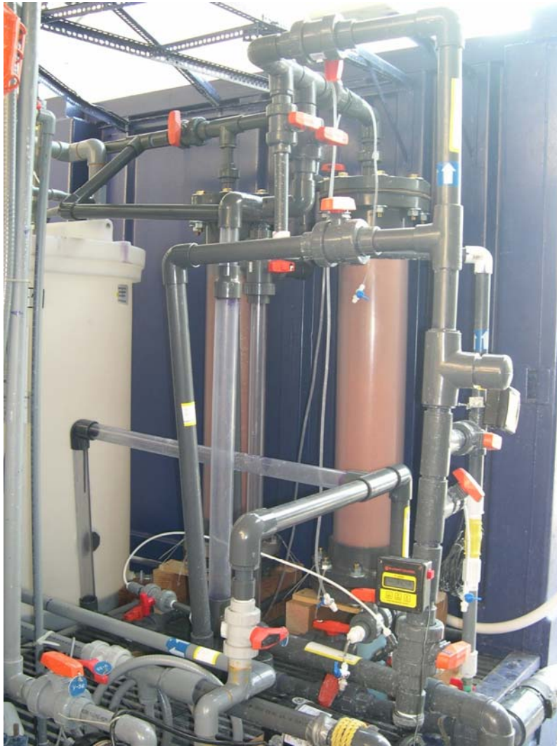
Figure 5. Ion-exchange subsystem of unit deployed at Baldwin Park
