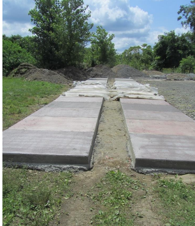
Figure 5.9 Panel groups D-E-F and G-H-I after formwork was removed with saturated covering
