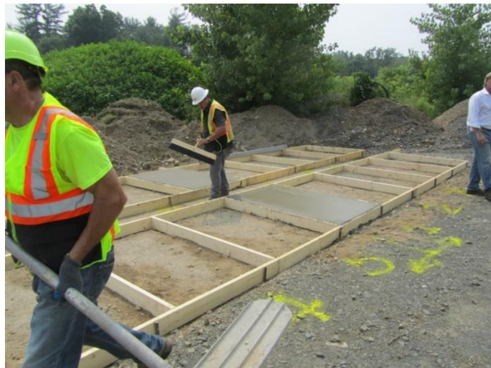
Figure 5.6 Worker using brush push broom to finish the surface of the panel
