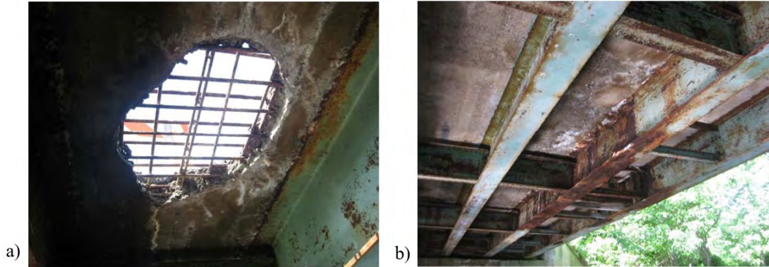
Figure 3.1: a) Hole through the deck and b) map cracking with heavy efflorescence at O-03-009 bridge (adopted from O03009-0TW-MUN-NBI)
