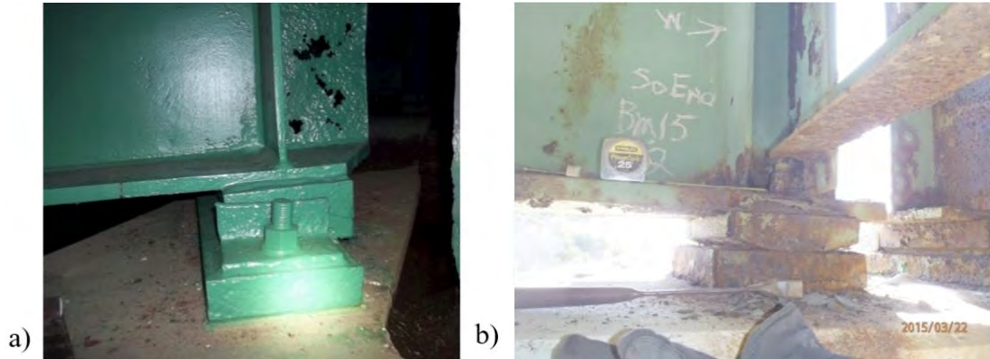
Figure 4.9: a) Expansion and b) fixed bearing types commonly found supporting corroded plate girders in Massachusetts
