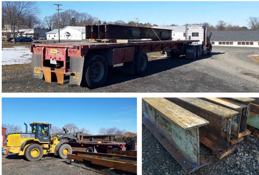
Figure 3.2: Delivery, unloading, and storage of first set of corroded beams
