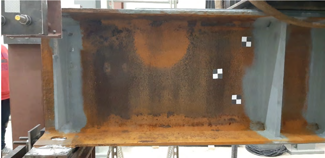
Figure 3.12: Corroded end of Specimen B
