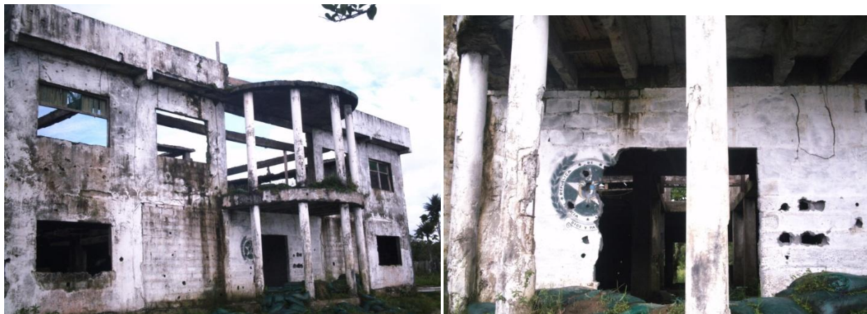
Figure 11: Destroyed Police Station II
