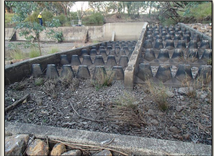
Reilly's Weir fishway on the Condamine River, Condamine, Queensland. Photo: Andrea Prior.
