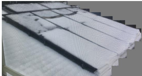
Figure 5: Lower roof under snow
